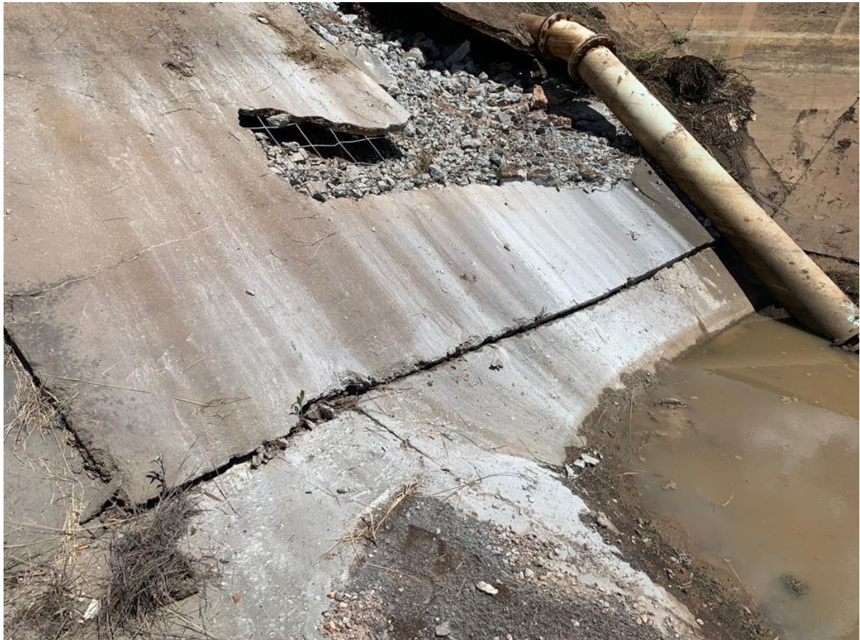
Picture 1: Damaged wall of water treatment plant in Koster before the KCC take over services.
