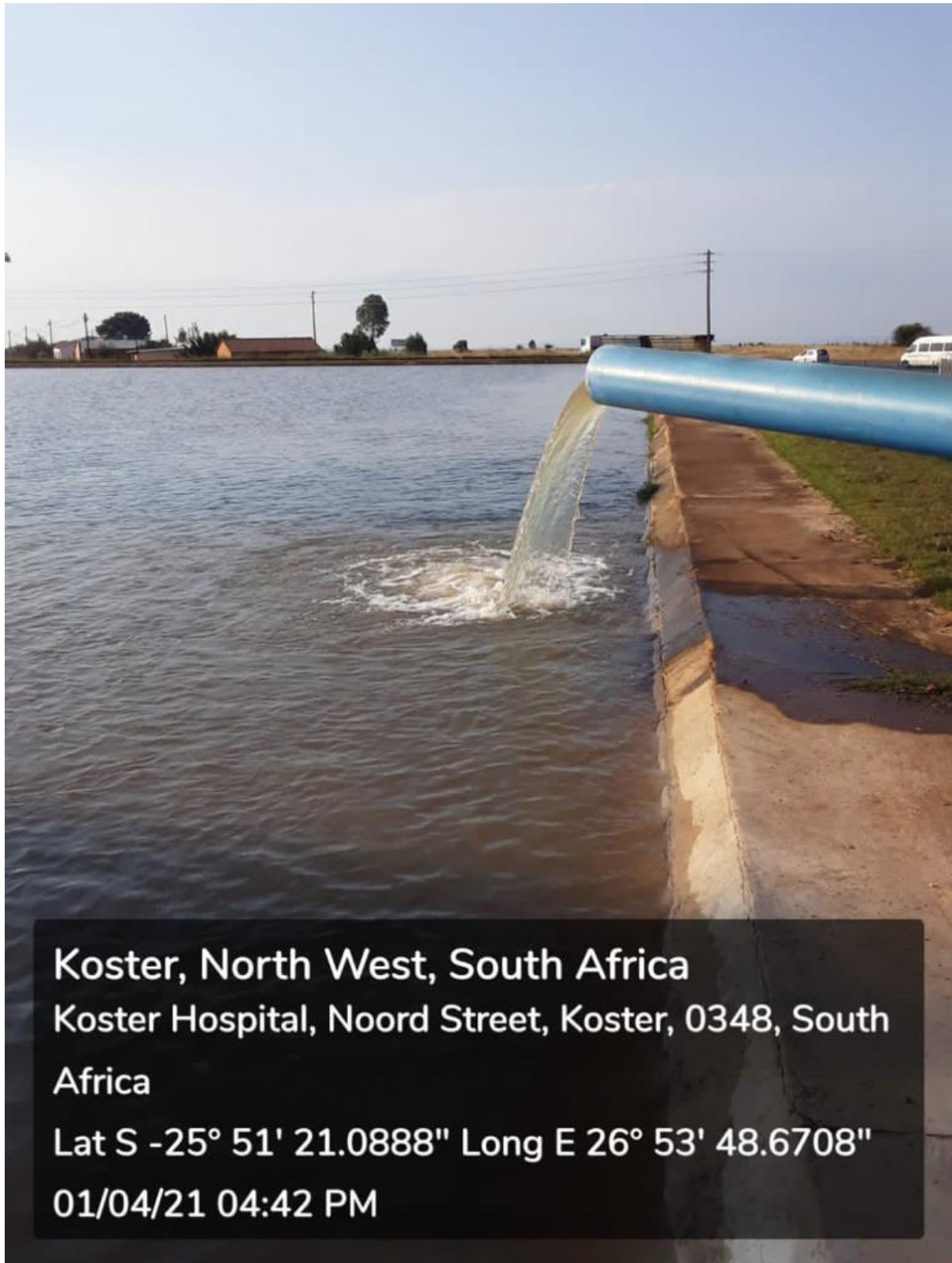
Picture 9: Water flowing to the water treatment plant in Koster.
