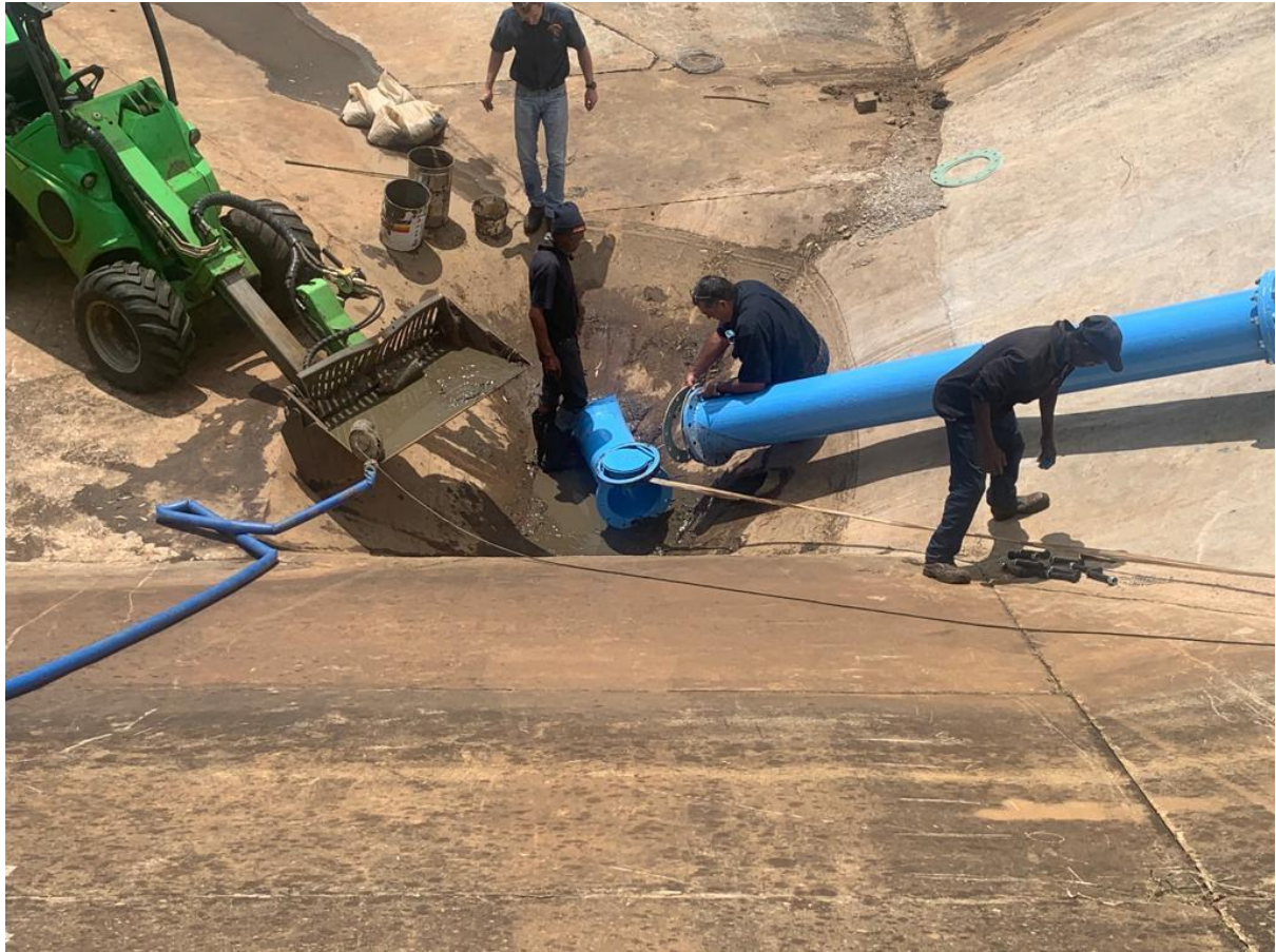
Picture 3: Repairs being done by member C of the KCC and his team to the water treatment plant in Koster.
