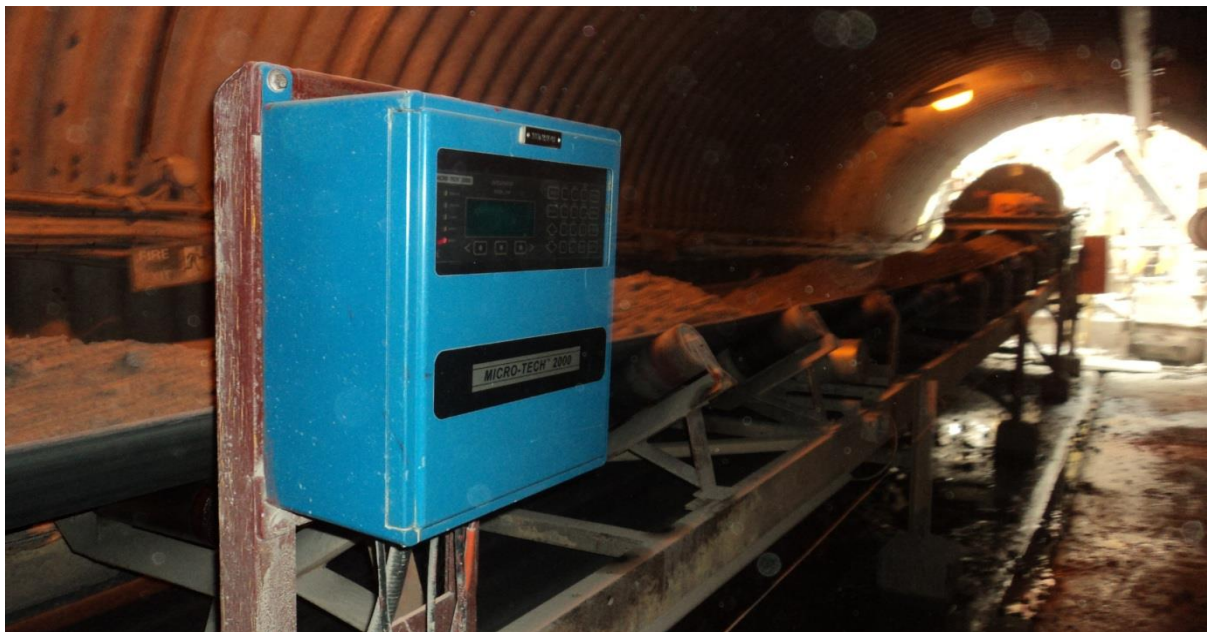
Figure 2.3 Electric weightmeter for mass measurement at plant (Iduapriem mine)
