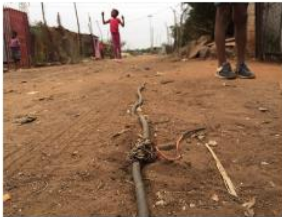
Fig. 2. Electrified wires loosely buried under soil in the street, branching to homesteads.
