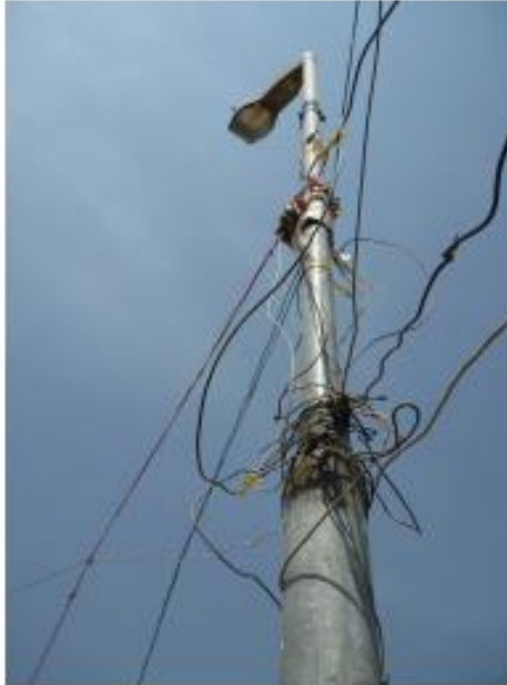
Fig. 1. Diverting power from street-lights using wires and tape.
