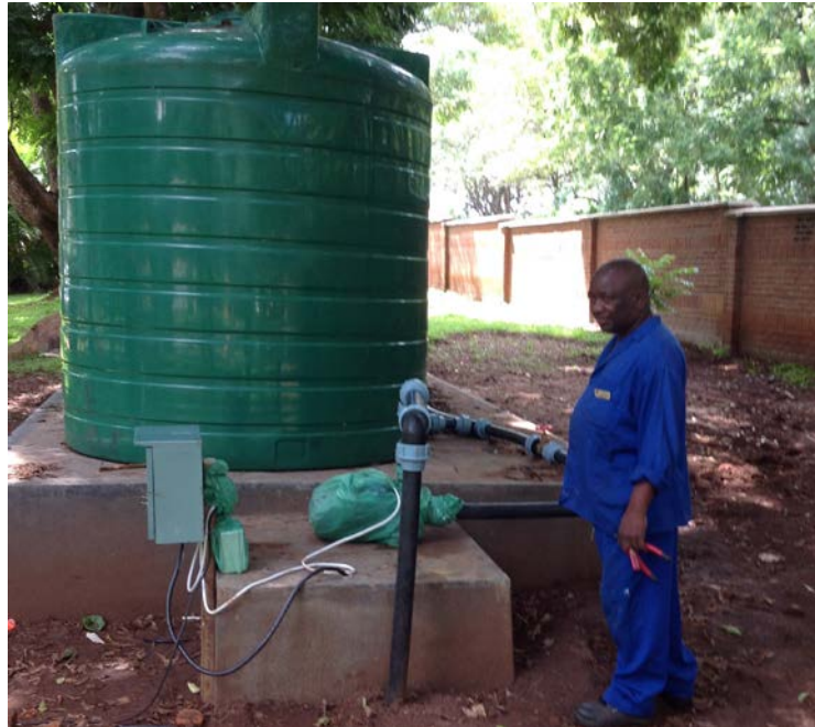
Figure 23: Borehole at Sunbird Capital Hotel Source: Author, Field Visits
