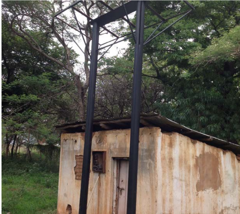
Figure 29: Solar Powered Borehole System
