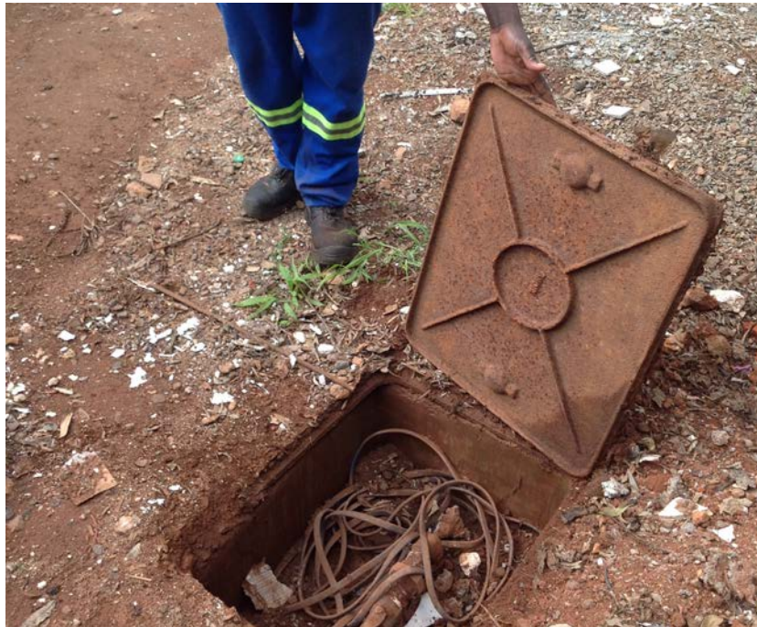
Figure 27: Sunken Borehole Pump System Source: Author, Field Visits
