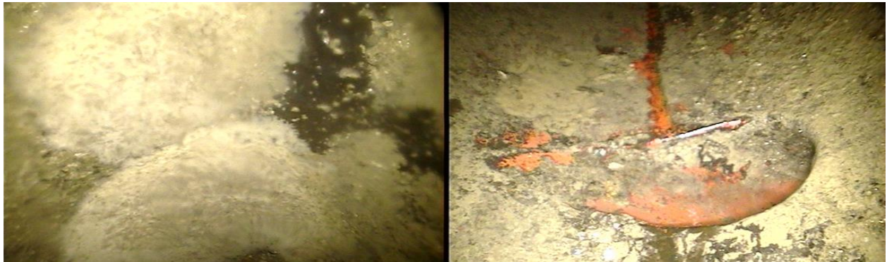
Figure 4-5: Photographic Evidence of Deposit Build-up at Air Valve Connection
