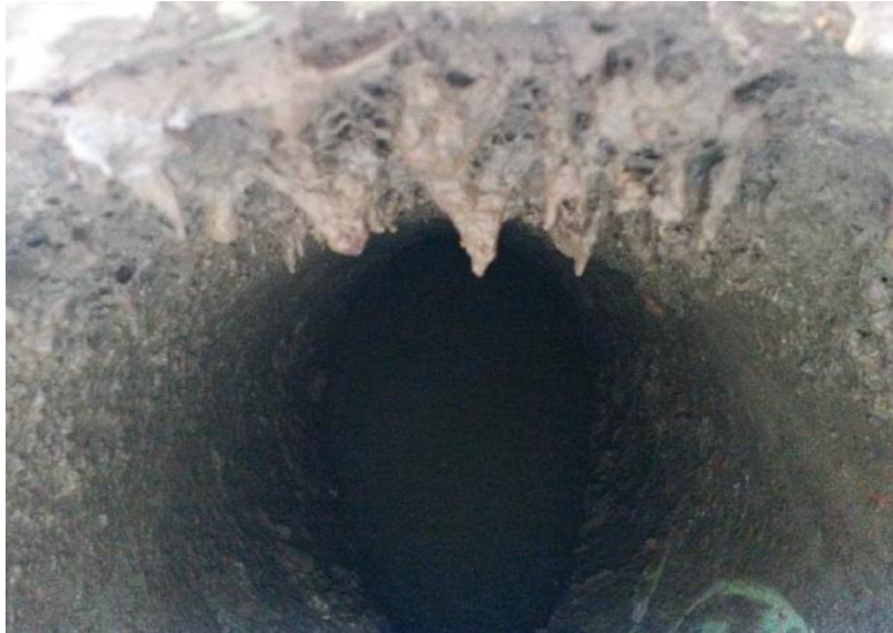
Figure 4-7: Deposit Build-up Inside the Old Pig Launcher Pipework
