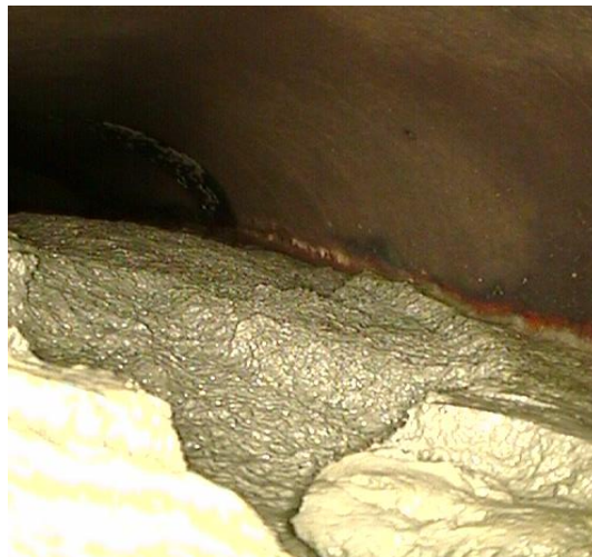
Figure 4-6: Photographic Evidence of Deposit Build-up (Accumulation of Deposits)
