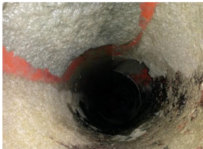
Figure 4-2: Evidence of Clay and Silt Build-up
