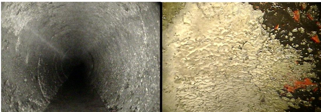
Figure 4-4: Photographic Evidence of Deposit Build-up
