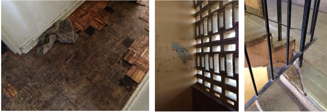
Figure 14: The dilapidated state of Jane's flat and the building as a whole.
