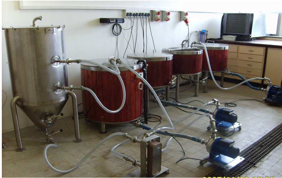
Fig 2.3. The Wits Microbrewery Plant-designed and supplied by Falcon Engineering (Pty) Ltd, South Africa.
