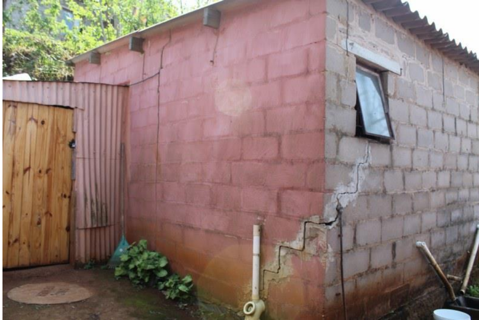
Image 1: Cracks in one of the houses in Waterloo Phase 5 (Source: Khubisa, 2017)
