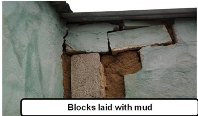
Cracks above windows with no lintels
