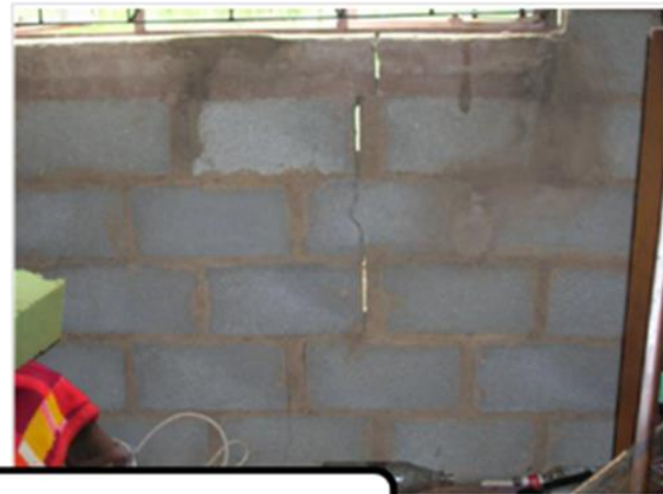
Cracks on wall
