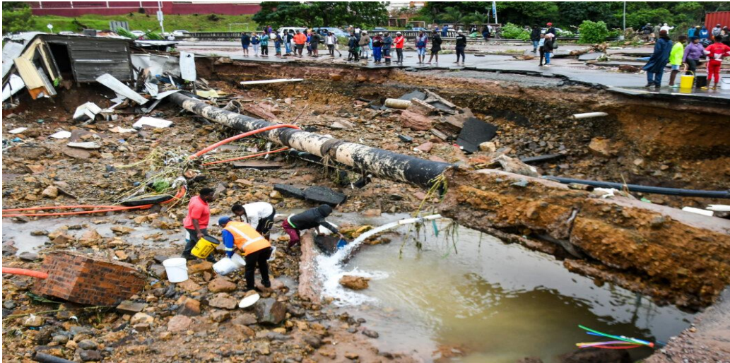
Figure 10: Damage to telecommunication fibre cables
