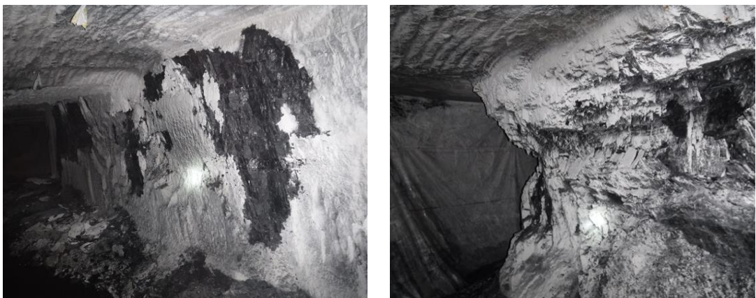
Figure 1-3: Excessive scaling and slabbing of the pillar corners and ribsides (sidewalls) due to increased vertical stress.
