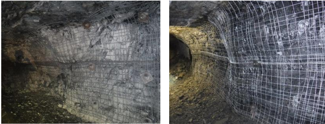
Figure 4-3: Pillars along Panel 1120 travelling road wrapped with mesh to prevent further scaling.
