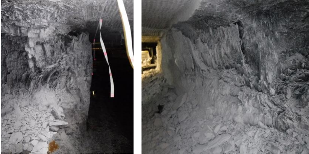
Figure 1-8: Excessive pillar scaling along Panel 1120 tractor road.
