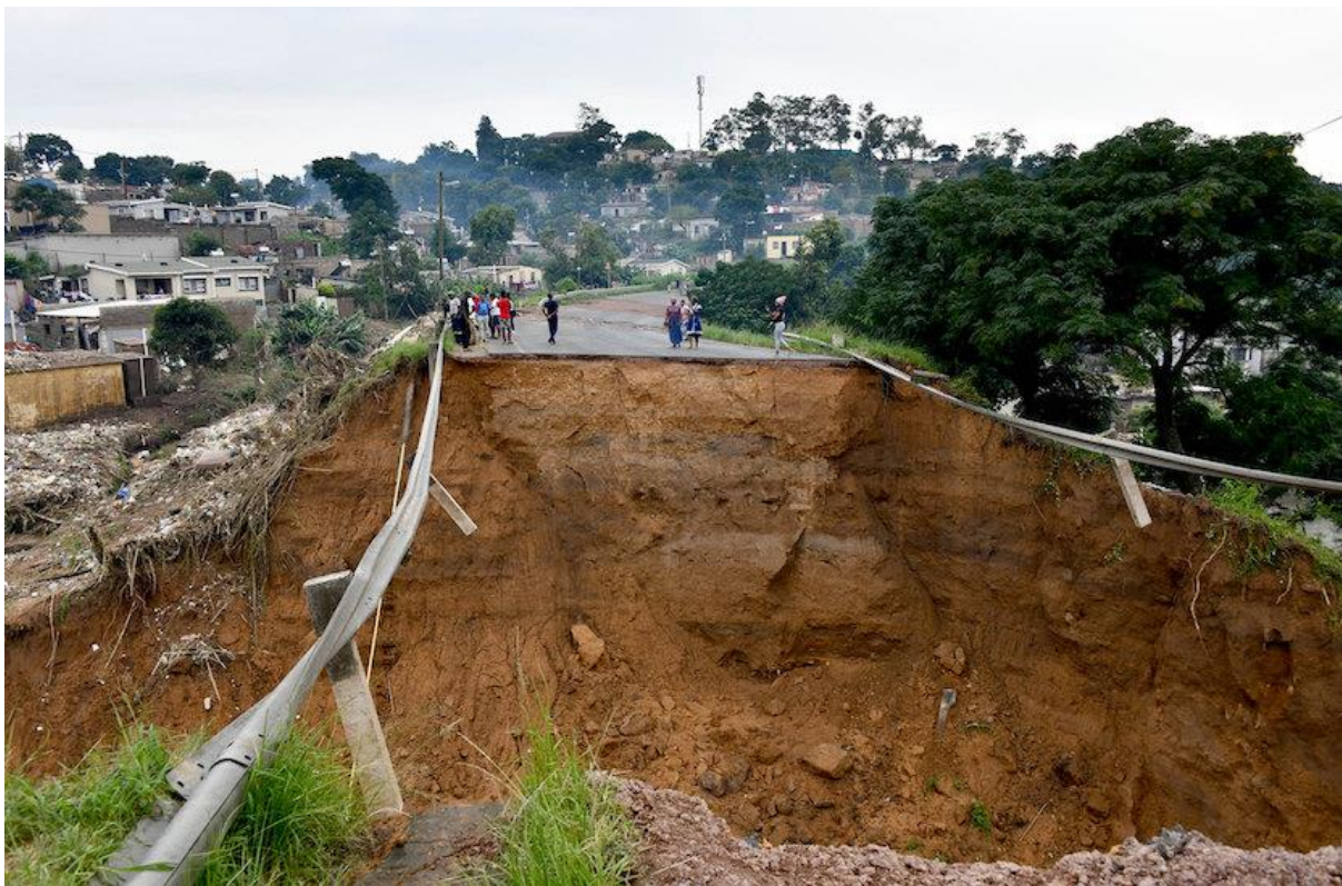
Figure 2.1: eThekweni flood damage in April 2022 (Magidimisha-Chipungu, 2022).
