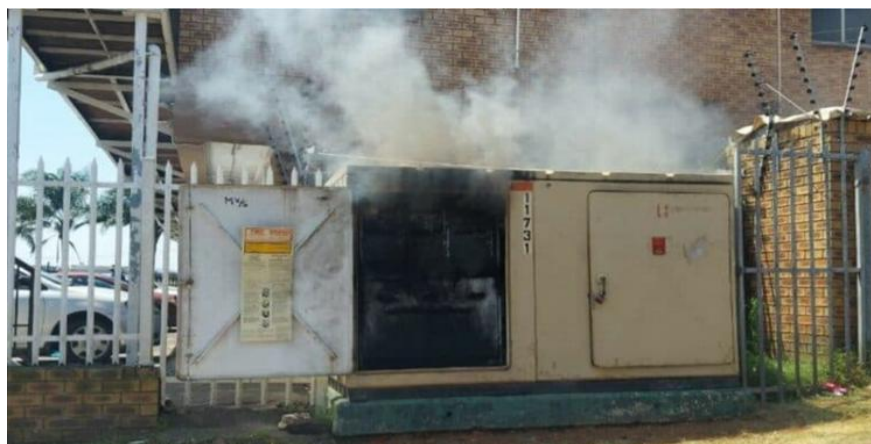
Figure 13: An example of electricity distribution infrastructure combusting due to extreme temperatures in the North of Durban, KwaZulu Natal (Habbib, 2025).
