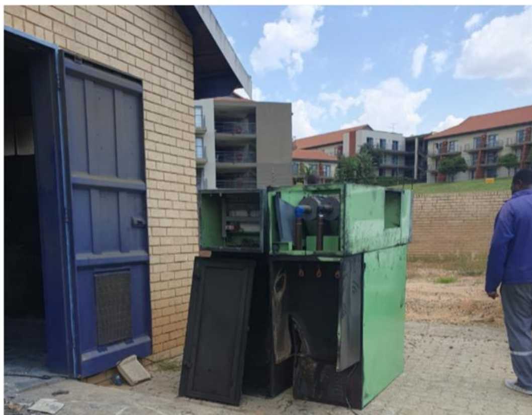
Figure 14: Substation switchgear after an explosion in the City of Johannesburg (Luvhengo, 2023).
