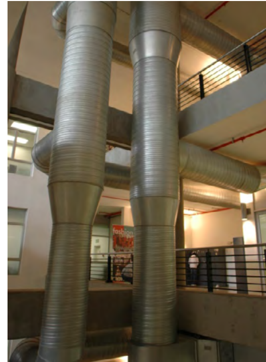
Figure 73: Exposed and oversized ventilation ducts cause noise pollution, UA (Author, 14.06.2009)
