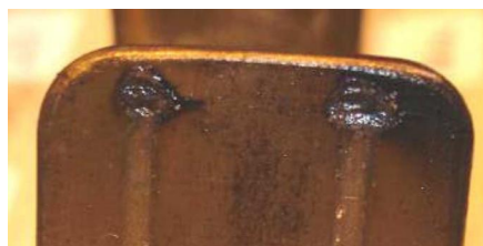
Figure 1.1 – Typical damage to changeover selector contacts [3]
