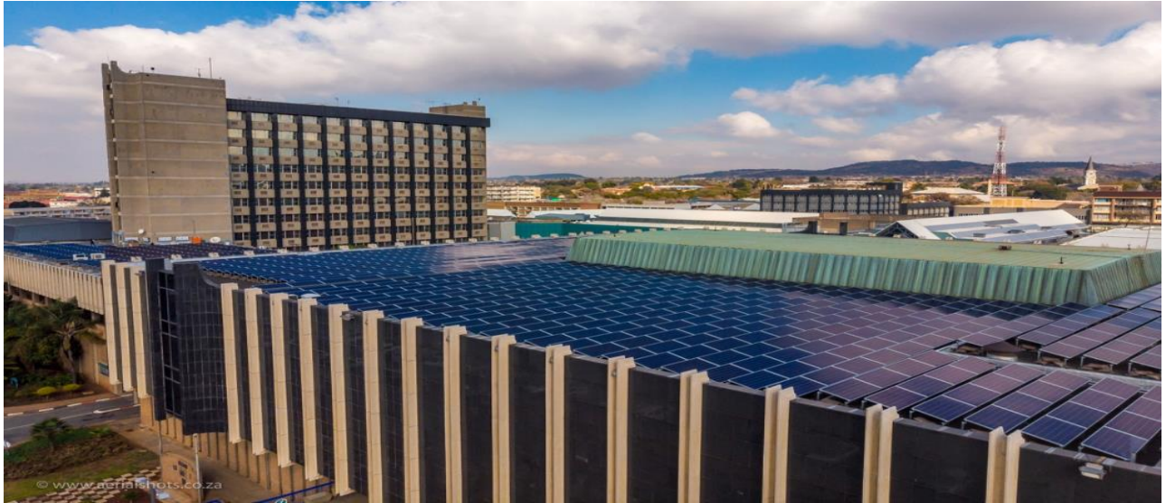
Figure 5.6: A closer caption of the Alberton Civic Centre rooftop PV, 500kWp system. 20 February 2018.
