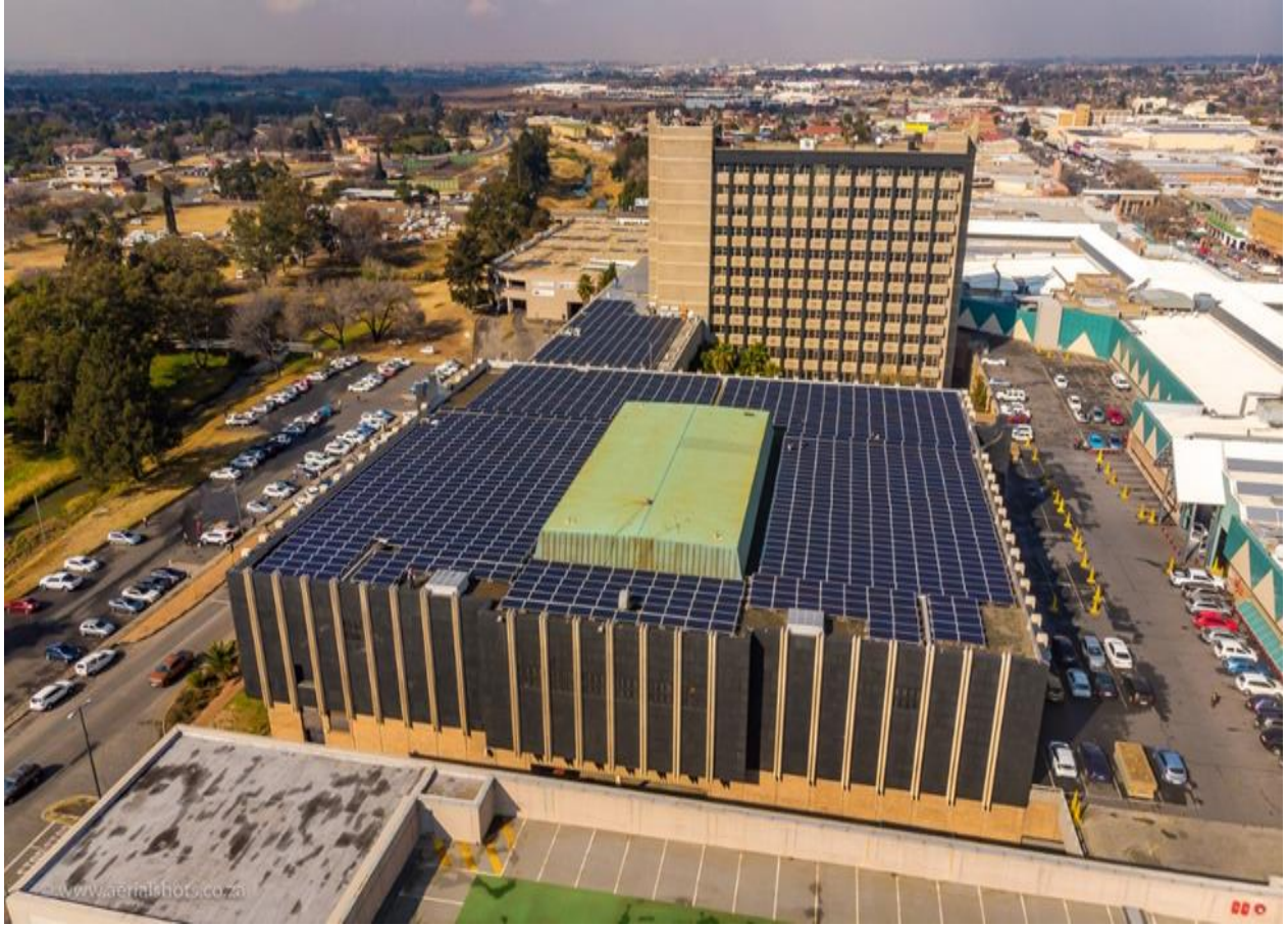
Figure 5.5: Rooftop PV, 500kW installed on the Alberton Civic Centre Ekurhuleni. 20 February 2018
