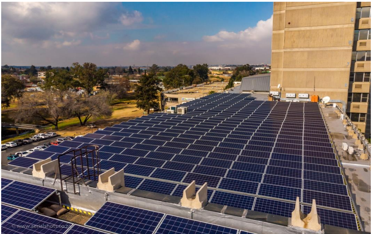
Figure 5.7: A different angle view of Alberton Civic Centre rooftop PV .20 February 2018.
