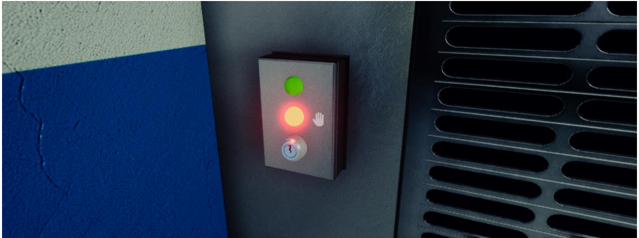
Figure 13. The red light on the gate control shows that the gate is locked.
