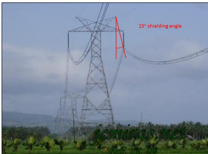
Figure 19: Structures of the Leyte - Luzon HVDC scheme in the Philippines 15 .
