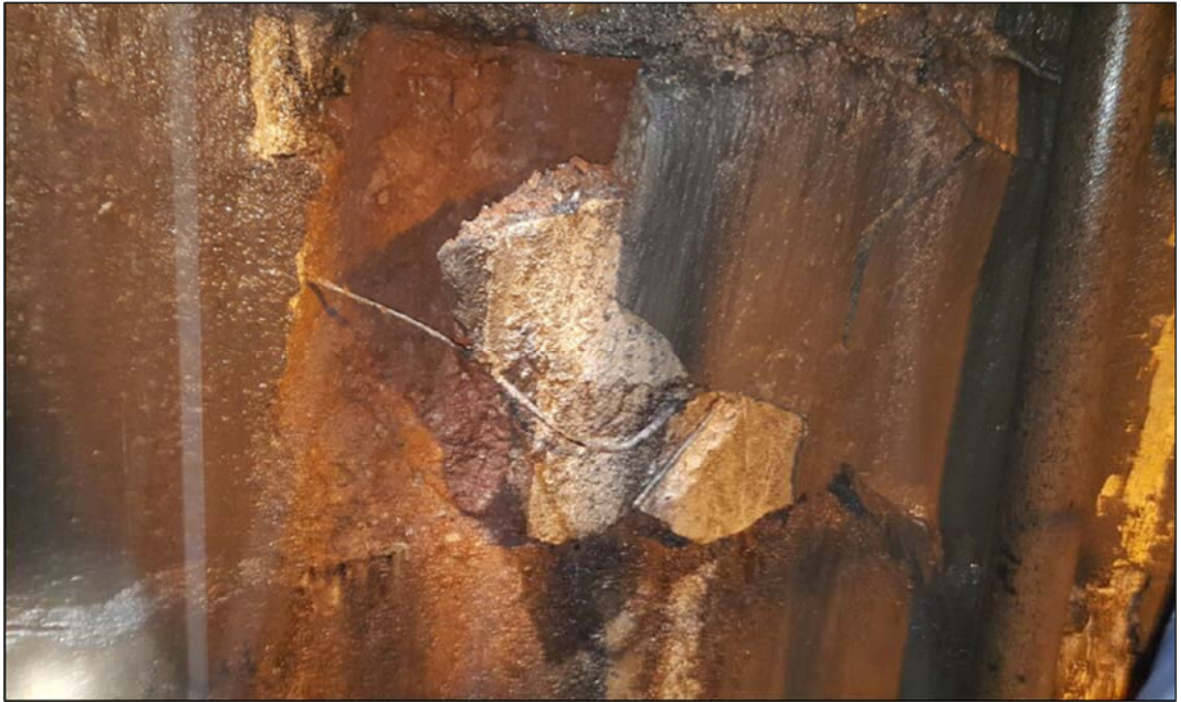
Figure 38: Shaft lining scaling off exposing the Red Clay
