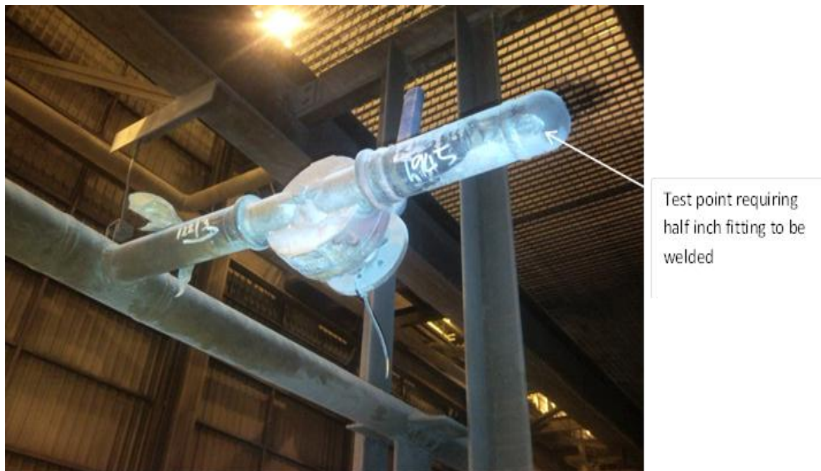
Figure 3-7: Test point on cold reheat drain line at forced dried Power Station A
