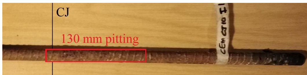
Figure 4.41: Corrosion in the 10 mm cover cold joint beams
