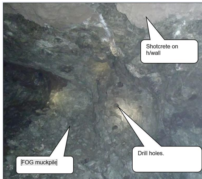
Figure 2-12. FOG from the Hex River fault zone (Sibanda, 2012)
