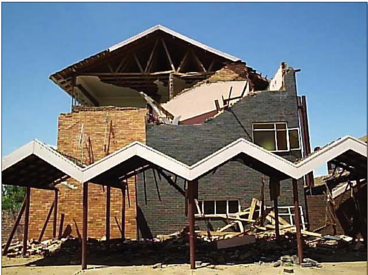
Figure 3.5: Damaged building at Stilfontein resulting from an earthquake event of magnitude, M_L = 5.3 on the 9th of March 2005 (Saunders et al. , 2008).
