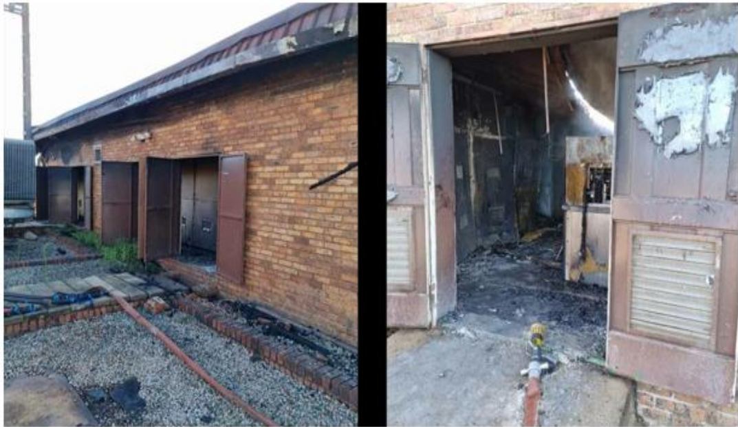
Figure 2: KwaThema substation 2022, source: CoE, 2024.
