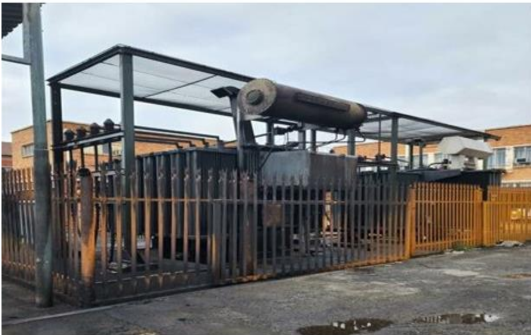
Figure 3: CoE Springs town substation in 2023, source: CoE, 2024.
