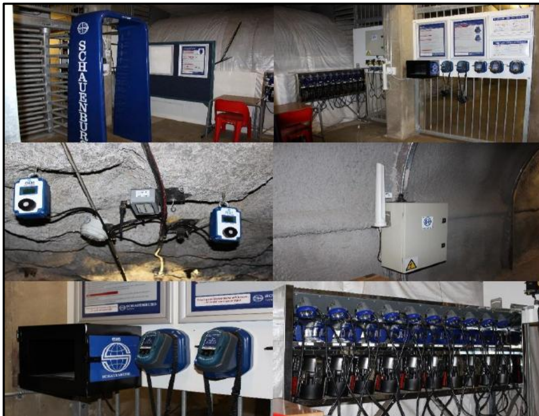
Figure 4-16 Schauenburg installation at WMI mock-up mine (Source: Faiq Javaid)
