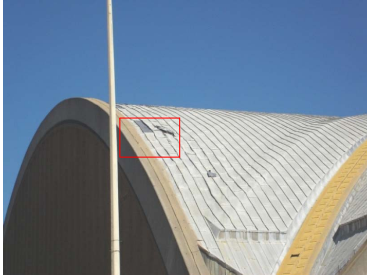
Figure 8.1- Local cladding damage observed on the Good Hope Centre
