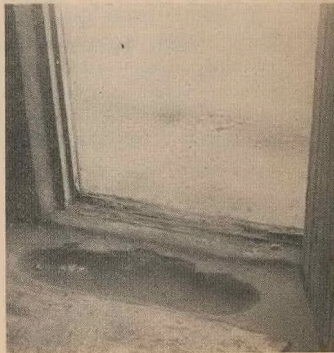
An ingenious method of drainage that has to be resorted to on account of the step down into the house.
