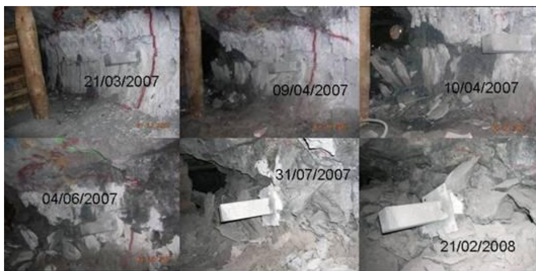
Figure 5-107 Union P1 fracture progression around the extensometer
