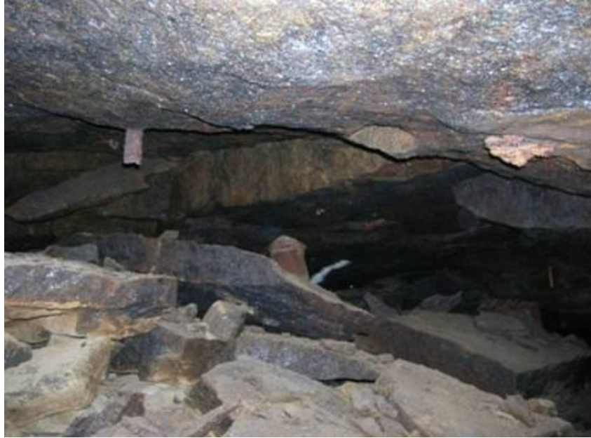
Figure 4-21 Impala site: FOGs adjacent to a pillar, resulting from horizontal fracturing in the hangingwall adjacent to the pillar
