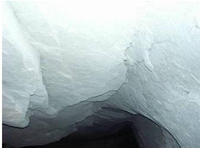
Figure 4-4 Horizontal stress fracturing observed in the hangingwall of a panel, adjacent to a pillar
