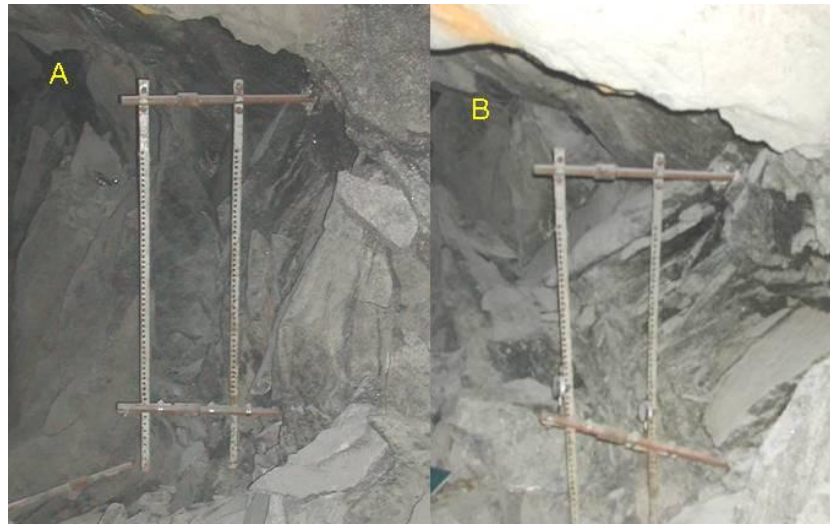
Figure 5-45 Amandelbult site: rotation of jumpers cemented into the centre of P2 near the top edge of the pillar and about 1 m vertically below. A = pillar failure, B = three months after pillar failure
