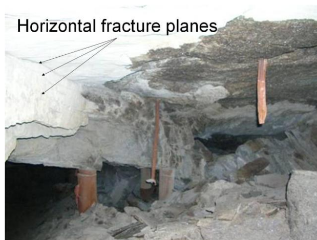
Figure 4-38 Impala site: horizontal fracture planes observed in the brow at the edge of the FOG in the face of Panel 8s
