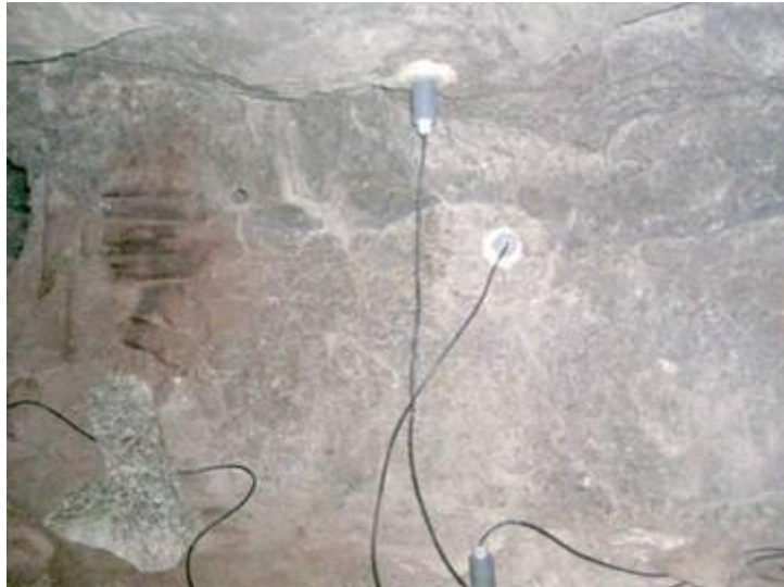
Figure 4-67 Impala site: abutment adjacent to the 7s face when this panel was isolated. The abutments near the face were almost unfractured
