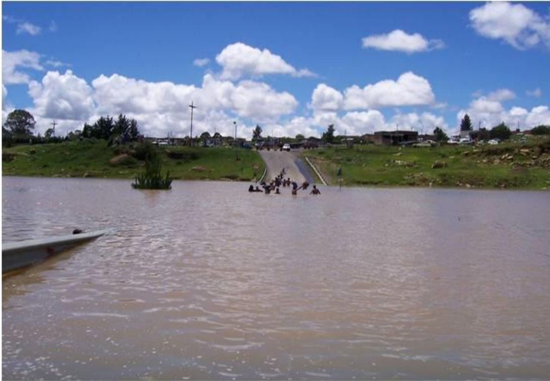
Figure 5.18: Road flooded in Motlejoeng, Mohale's Hoek, disrupting movement of people and goods in January 2011.
