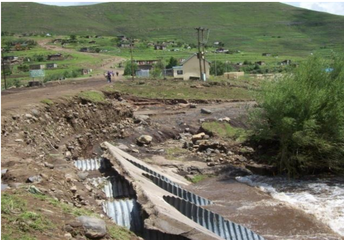
Figure 5.17: Bridges and roads washed away in Mpharane, Mohale's Hoek during heavy rains (Jan 2011). Source: Own photo
