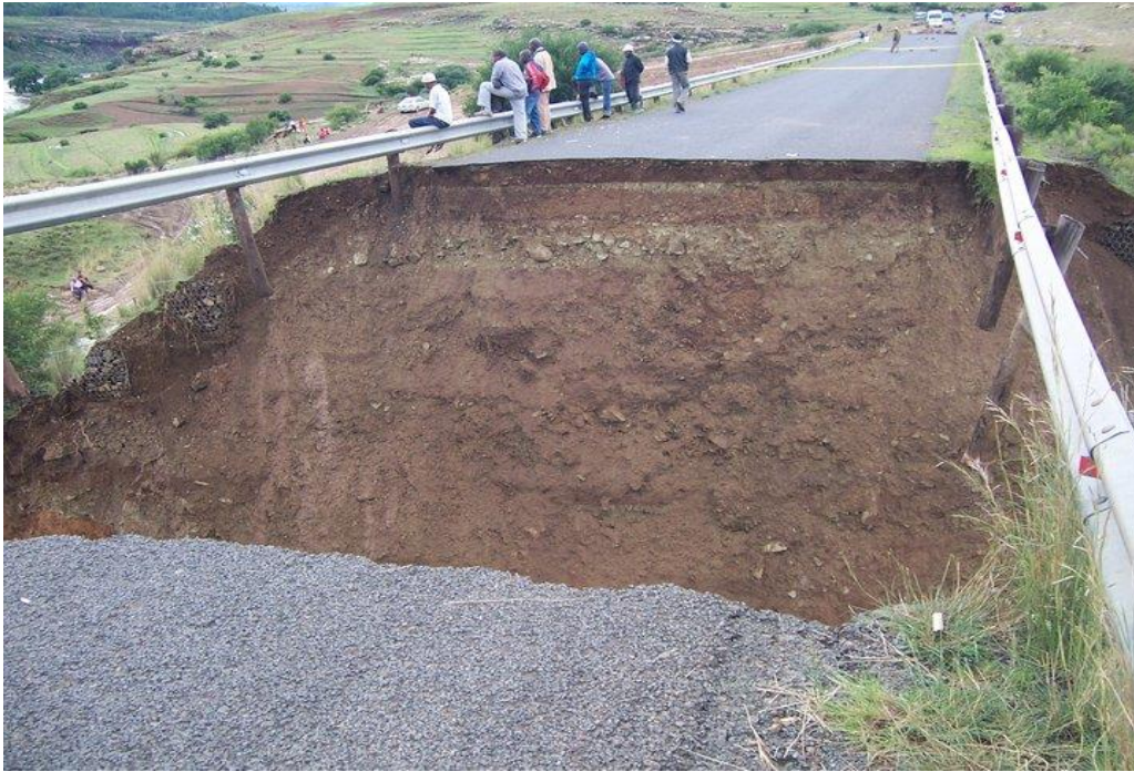
Figure 5.15: Bridge washed away in Ha Selaitara, Quthing during heavy rains (Jan 2011). Source: Own photo
