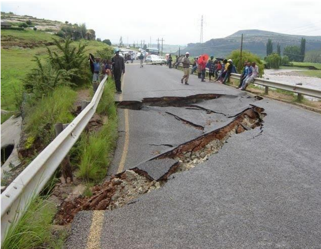
Figure 5.19: A road destroyed by floods in Mashaleng, Mohale's Hoek in January 2011. Source: Own photo
