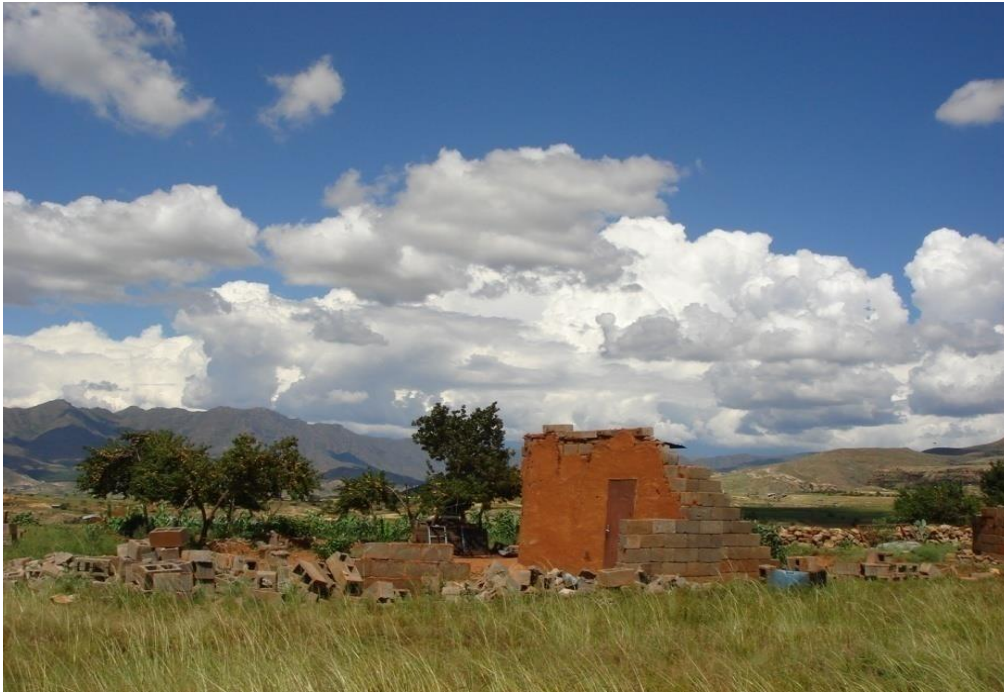
Figure 5.39: A house completely destroyed by wind at Moyeni, Quthing (January, 2010). Source: Own photo
