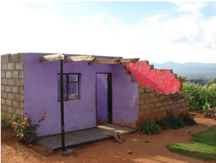
Figure 5.40: Roof blown off by wind in Mohale's Hoek (January, 2010). Source: Own photo
