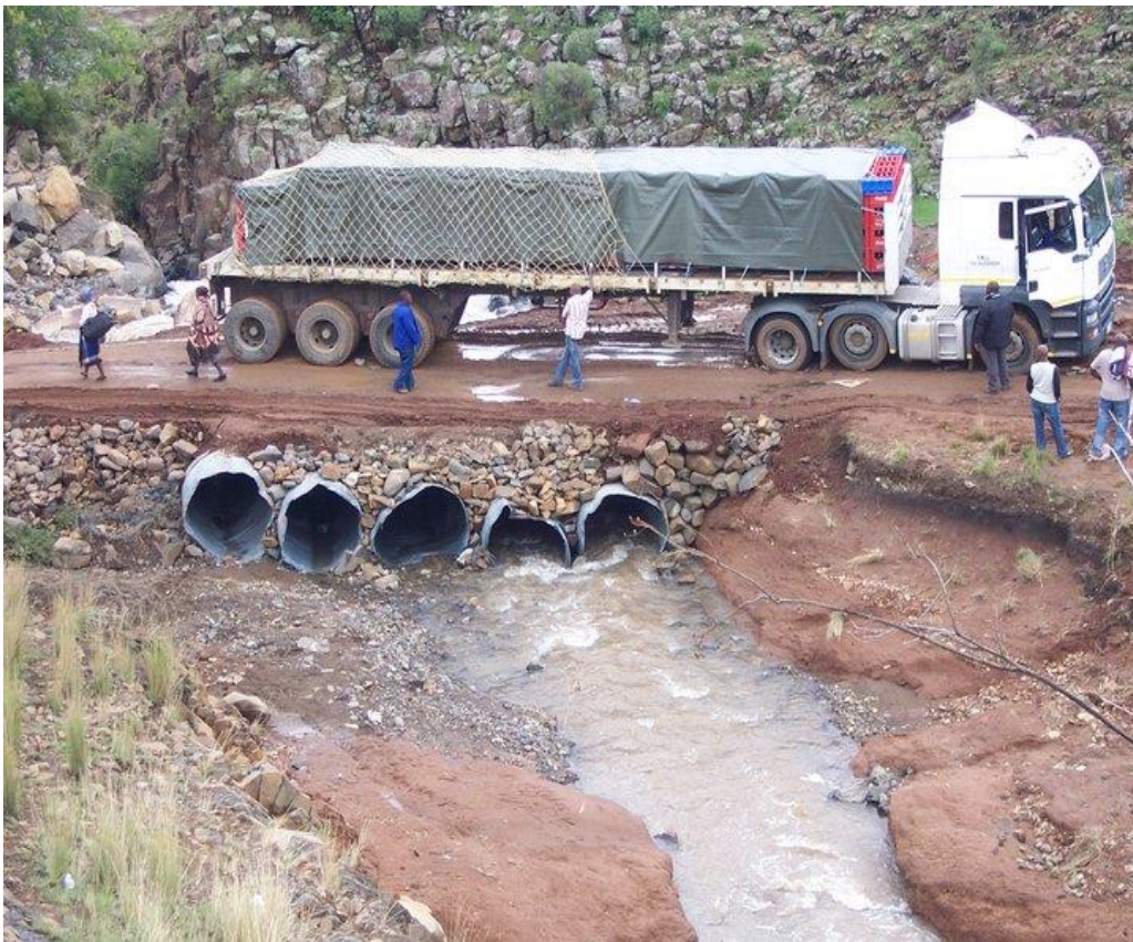
Figure 5.16: A make- shift road/bridge in Ha Selaitara, Quthing after heavy rains (Jan 2011). Source: Own photo
