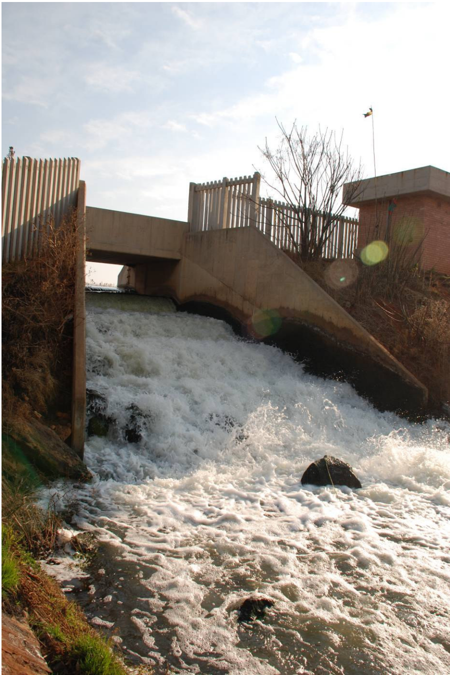
Figure 3.4.1: Discharge point of the Olifantsvlei sewage treatment plant ponds into the Klip River Wetland (August 2008).
