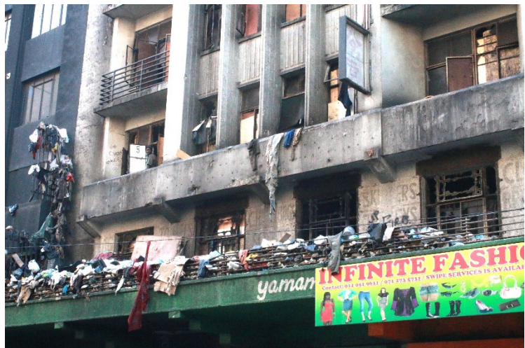
Figure 1: Dilapidated Building in Johannesburg's Inner-City UDZ
