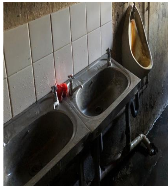
Picture 22: Image showing basin and a urinal
