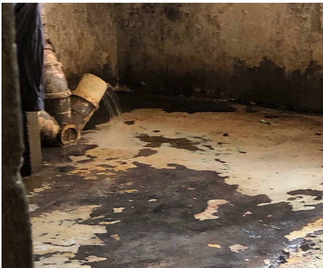
Picture 24: An image of water gushing out in one of the bathrooms at Jeppe hostel. (Source: Own)
