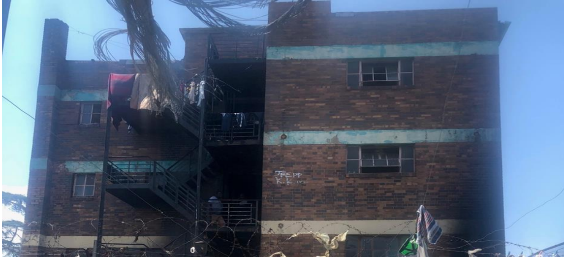
Picture 23: Image of a block with illegal electricity connections (Source Own)
