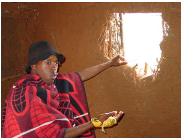
Hole in the wall where somebody broke into the shop
