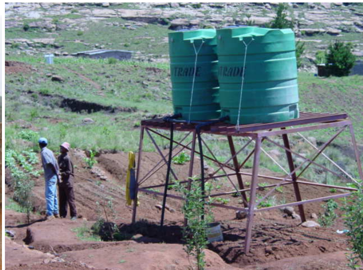
The gravity fed tanks installed below the dam provide a means for irrigating the garden
