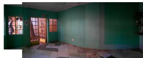
Transformed garage in need for 'as built' permit
