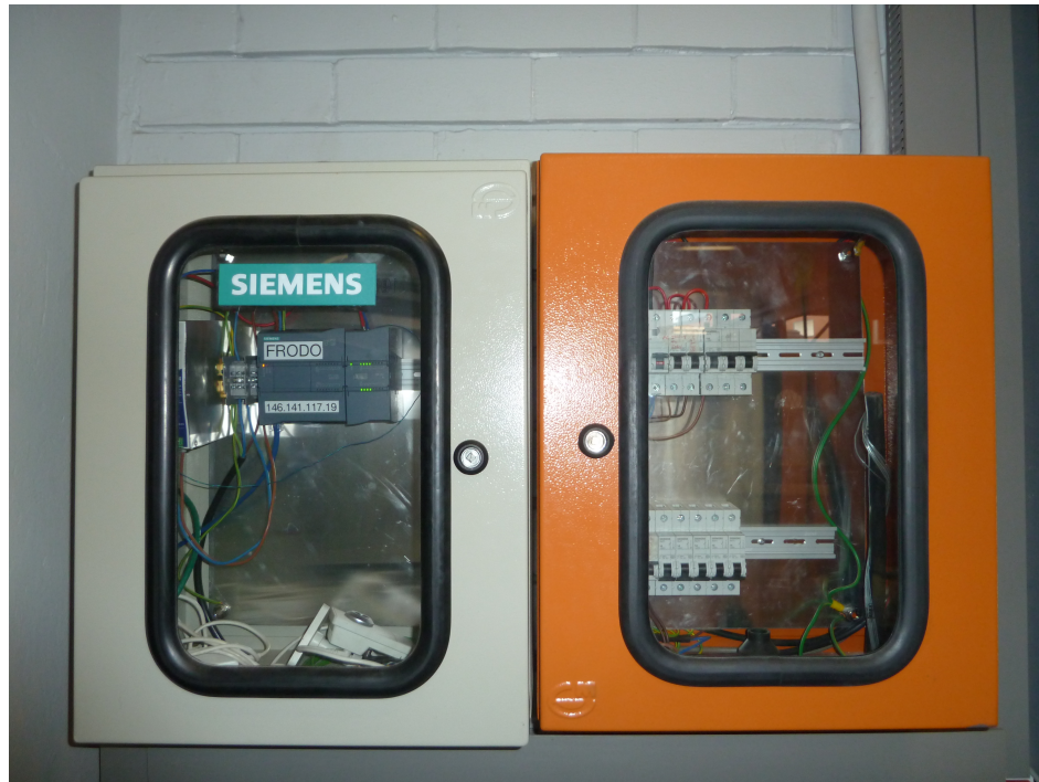
FIGURE A.6: Electrical distribution box and inverter.
