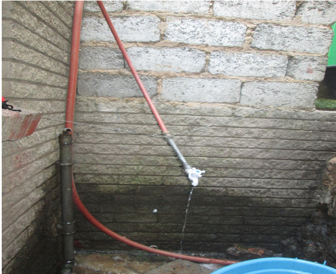
Shared Warehouse Illegal Water Connection
