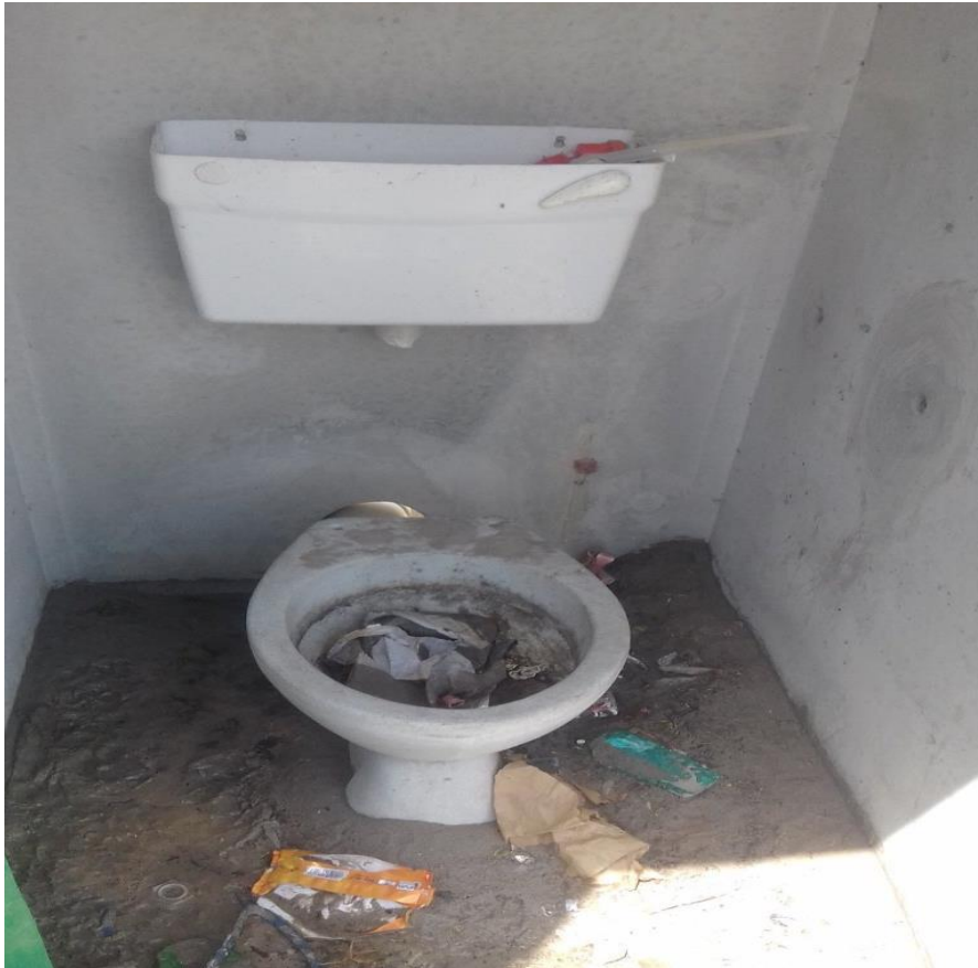
Dirty and Broken Communal Toilet
