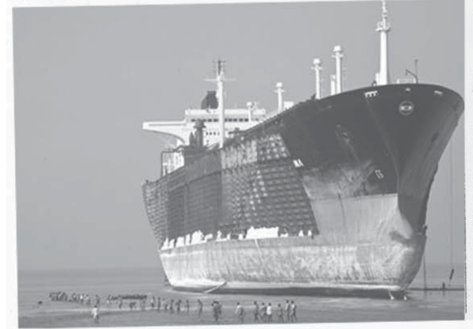
Everything is recycled as workers in the ship breaking industry dismantle oil tankers by hand, under dangerous conditions. Photograph: Andrew Holbrooke/Corbis
