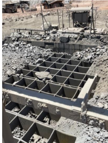
Figure 3.7: Site Run of Mine (ROM) tip for initial ore unloading
