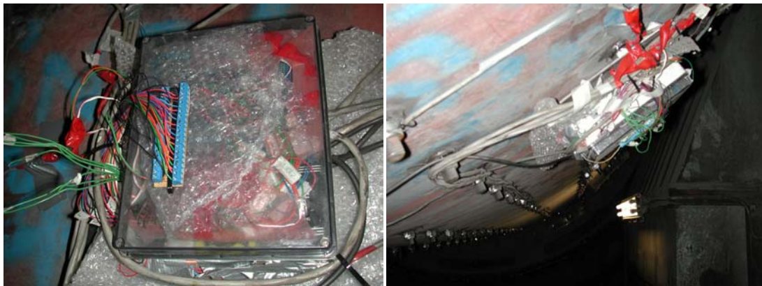
Figure A3.2.4: Control box mounted to steel base plate and onto mill shell. Bubble wrap was used between the steel base plate and control box to absorb vibrations from the mill shell.
