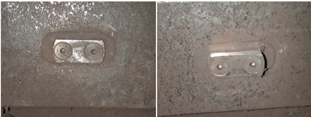
Figure A3.2.2: Installed conductivity probes CM1 (left) and OCM1 (right) as viewed from inside the mill. Pictures indicate the 3mm and 9mm height difference above the liner between CM1 and OCM1, respectively.
