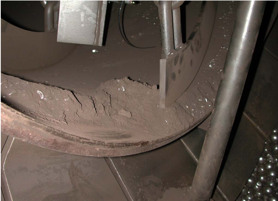
Figure 3.8: Picture of screw conveyor taken from inside the mill shell (mill rotates in an anti-clockwise direction). Picture indicates the approximately 15mm thick layer of coal dust present inside the mill.
