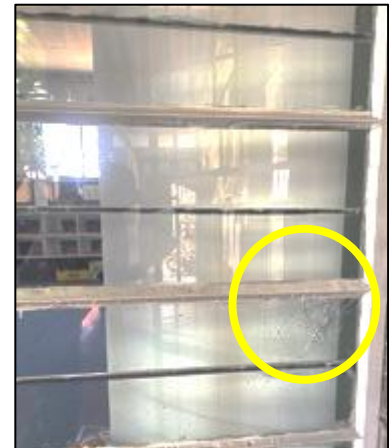
Figure 11: Stray bullet hole in the window of FE4's business premises
