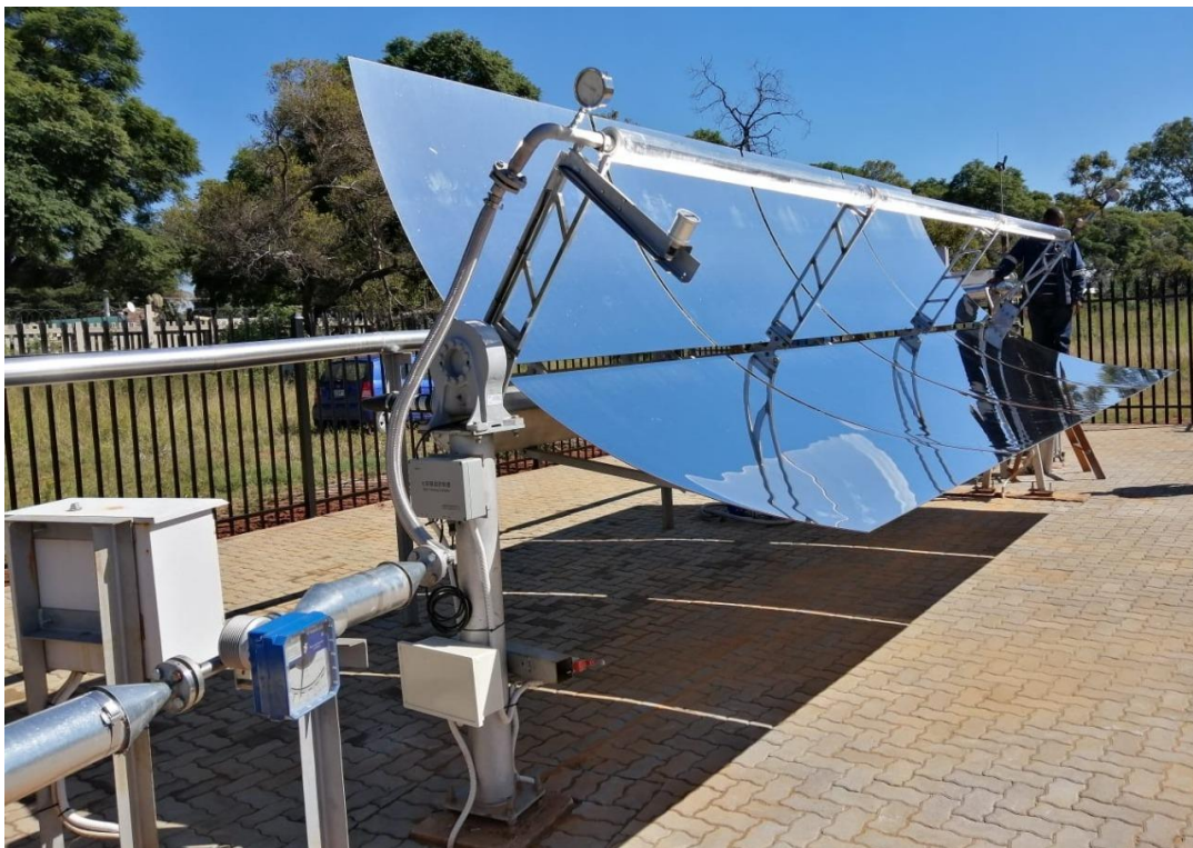
Figure 3.8. Parabolic trough (PT20) installed at ARC-AE premises
