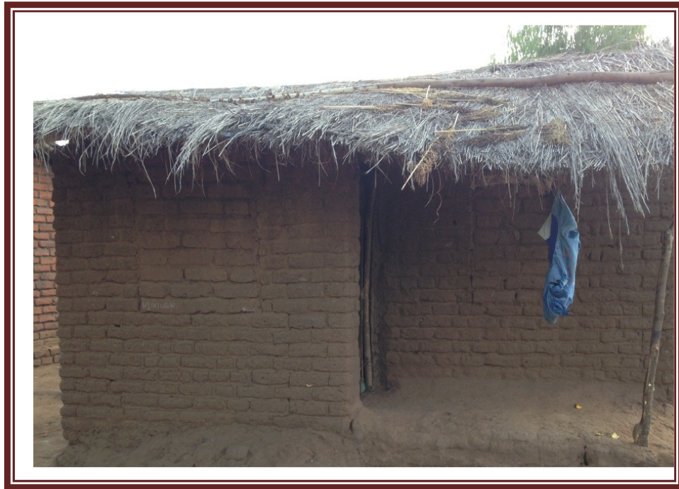
Figure 25: Dilapidated house where the elderly live
