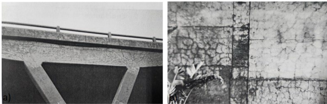
Figure 2-14: a) Elements of a bridge deck displaying distress in the form of severe map-cracking b) Wall displaying distress in the form of severe map-cracking (Blight and Alexander, 2011)
