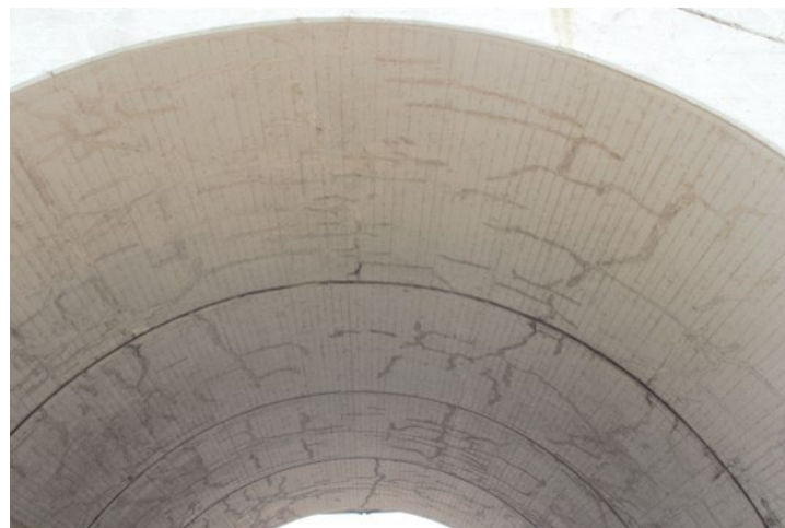
Figure 4-6: Extensive map-cracking on the underside of “sheltered” arch surfaces
