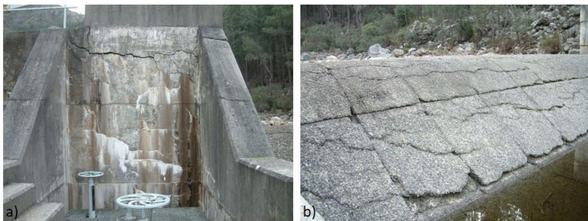
Figure 2-8: a) ASR gel and severe cracks present on the sidewall of the outlet works b) Severe cracks present on the weir wall (Courtesy of Y.Ballim)
