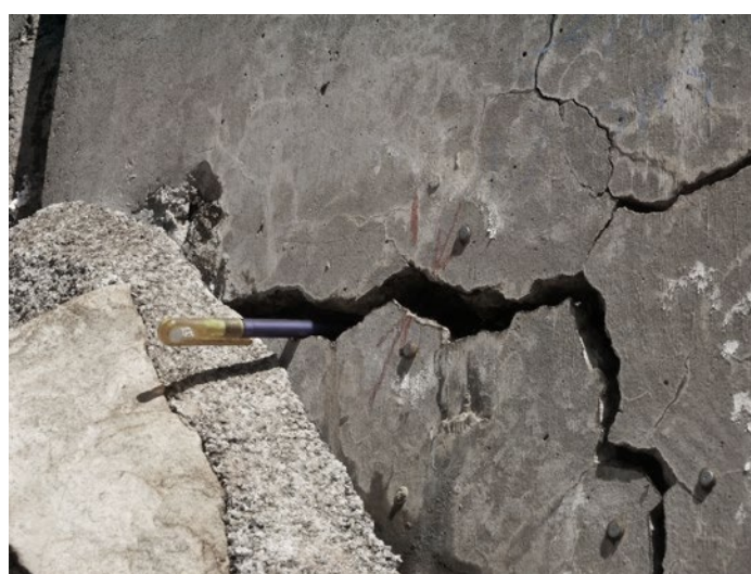
Figure 2-9: Strain measurement of crack width openings taken periodically to monitor the progress of ASR deterioration on the East side, South Abutment, of the M1 Empire Road Bridge. (Courtesy of Y. Ballim)
