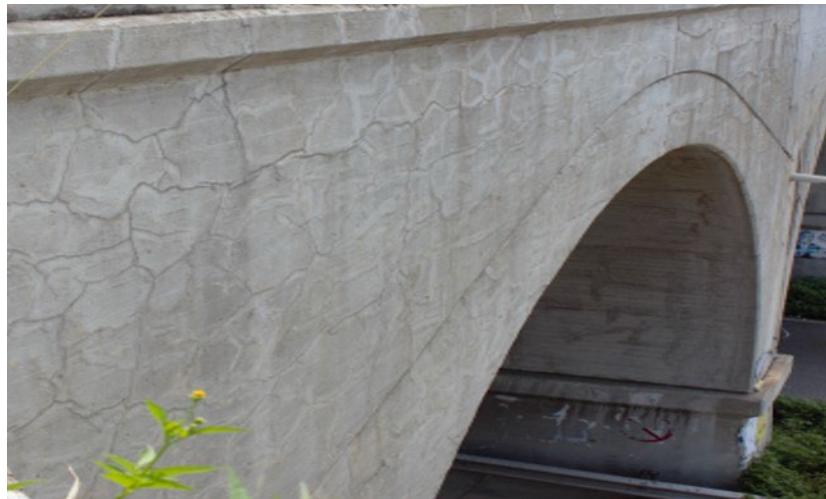
Figure 4-5: Evidence of map-cracking on the South facing exterior of RC railway bridge
