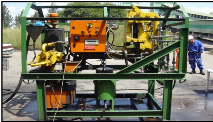
Figure 19: The Technicas Hidraulicas (TH) pilot plant filter press.
