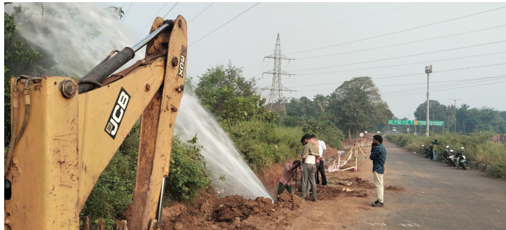
Figure 1.1: Water pipeline damaged as a result of roadworks - sourced from The Goan Network
