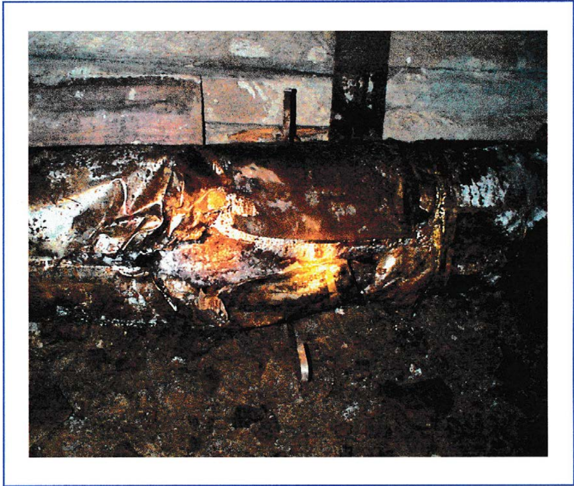
Figure 4.7 Damaged chilled water pipe insulation system (Source Rawlins, 1998)
