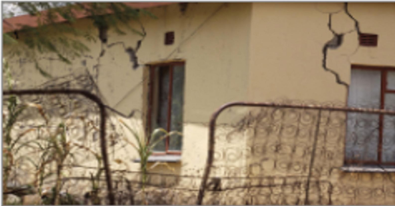
Picture of crack in house
