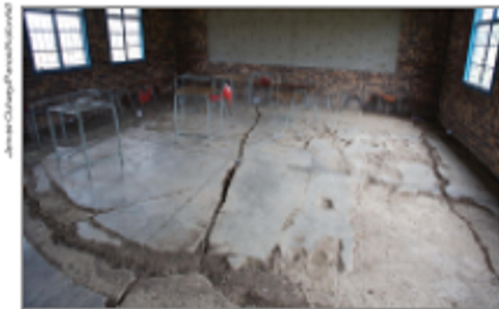
Picture of crack in school classroom floor
