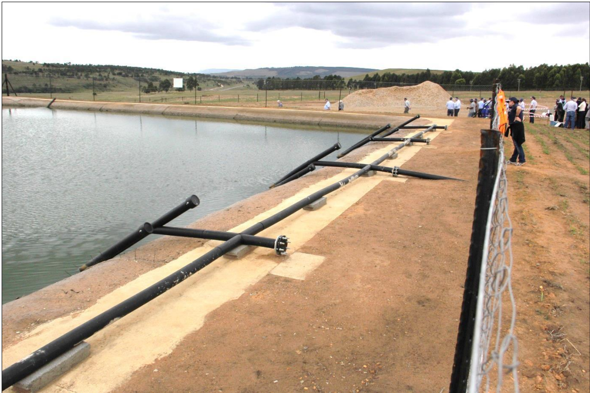
Figure 12: Constructed DPBR with inlet manifold pipes (Pulles & Meyer, 2012)
