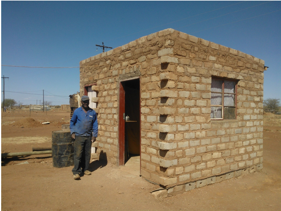
Photograph 14: Mr Siphon Plaatjies standing next to the first phase of his newly built house. Behind him is the room he lets out for rental income.
