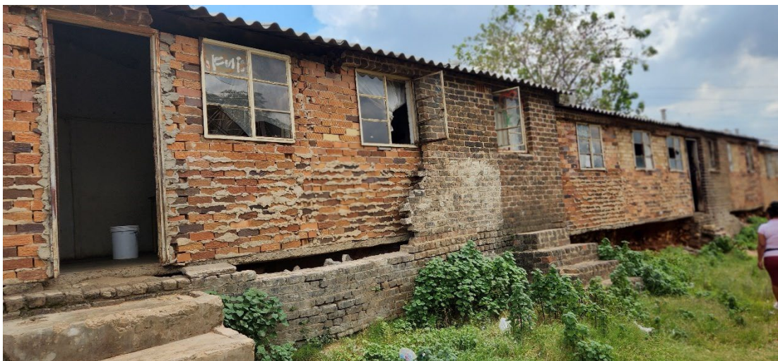
Figure14: The Diepkloof hostel's foundation is collapsing.
