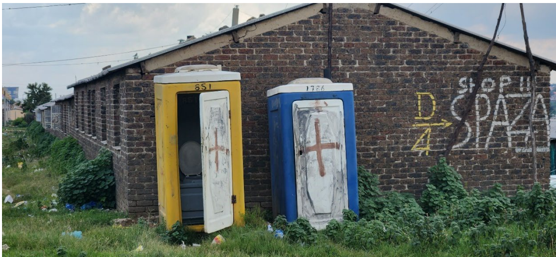
Figure 13: Communal toilets at the Diepkloof hostel
