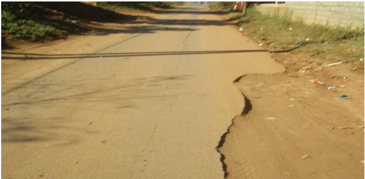
Figure 2.3: The State of the Road Linking Parts of Eteni and Matsapha Main Road
